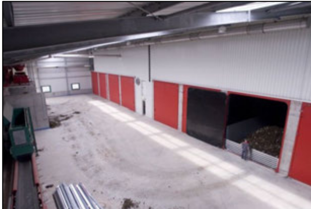
Mixing Hall and Anaerobic Digestion Tunnels
