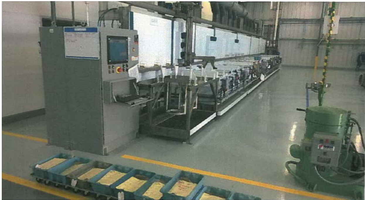
Figure 1: The newly installed plating line
