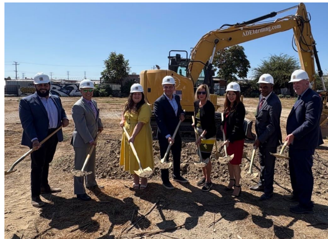
Awarded CDLAC bonds and 4% LIHTCs in December 2024, Amanda Villas in Southeast Los Angeles County broke ground in fall 2025. It will offer 140 apartment homes for seniors earning below 50% AMI and will feature a state-of-the-art health center, which will provide comprehensive medical, dental and behavioral health services to all residents. It is scheduled to open in Winter 2027.
